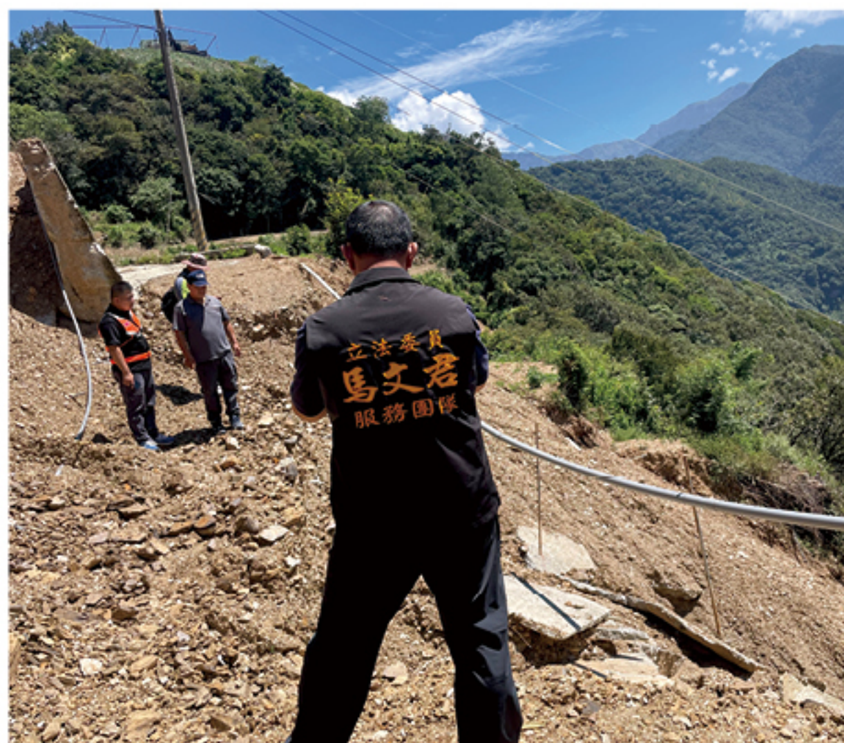
邊坡分工整治會勘
