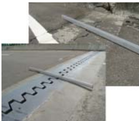
圖4.56 伸縮縫安裝比路面高出或太低
