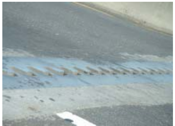
圖4.12 齒型伸縮縫進橋側翹起
