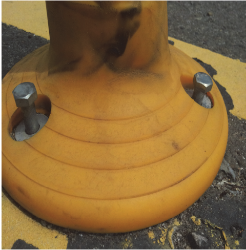
(a)螺栓固定不確實
