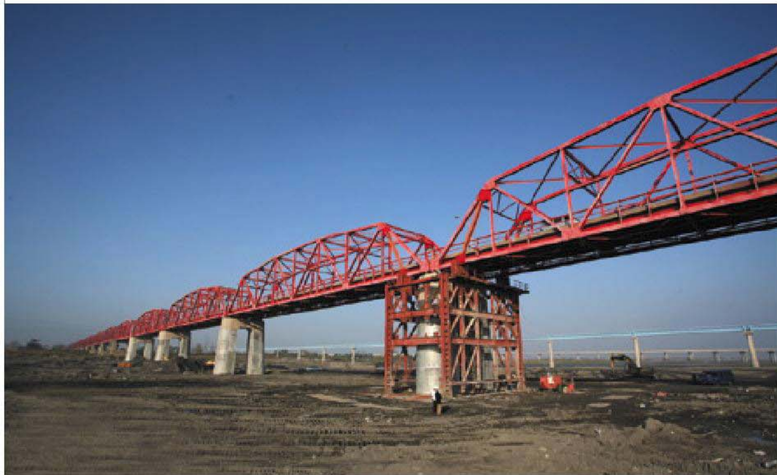
145線西螺大橋—橋墩換底工程 County Highway No.145 Siluo Bridge's base of piers reconstruction
