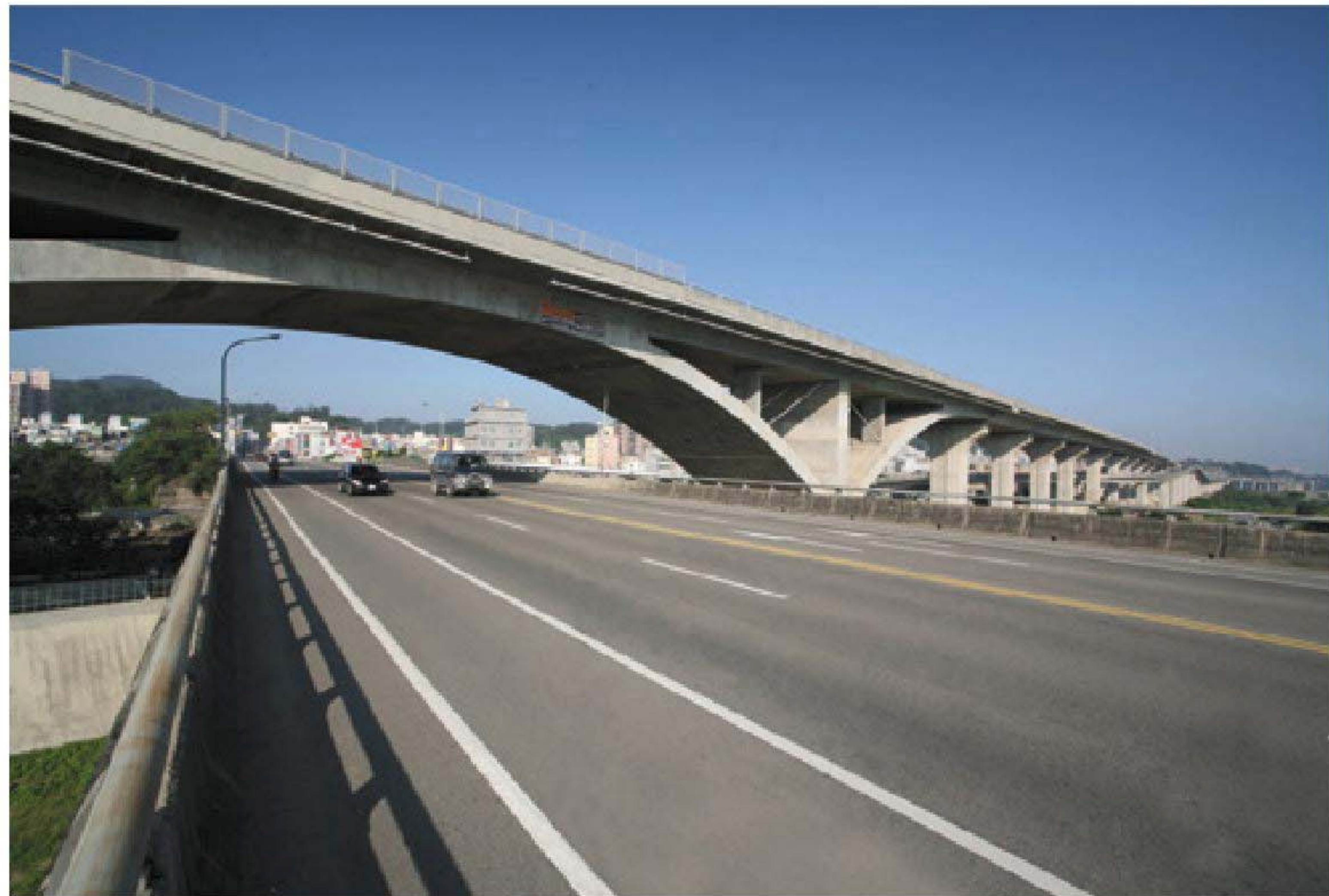
18 臺68線跨越123線竹林大橋 Taiwan Provincial Highway No.68 to overpass the County Highway No.123 Cross Zhulin Bridge
