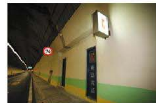
八卦山隧道行控中心機房 Baguashan Tunnel Operation Control Center equipment room
