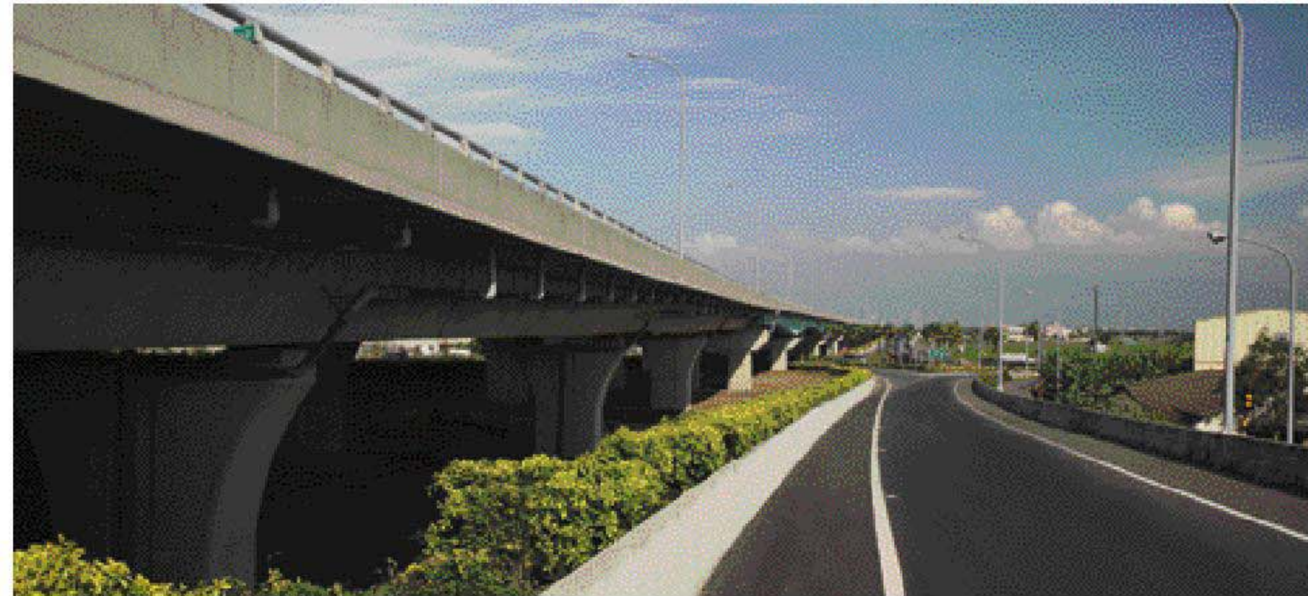
土庫虎尾交流道 (臺78線/145線) Tuku Huwei Interchange (Taiwan Provincial Highway No.78 / County Highway No.145)
