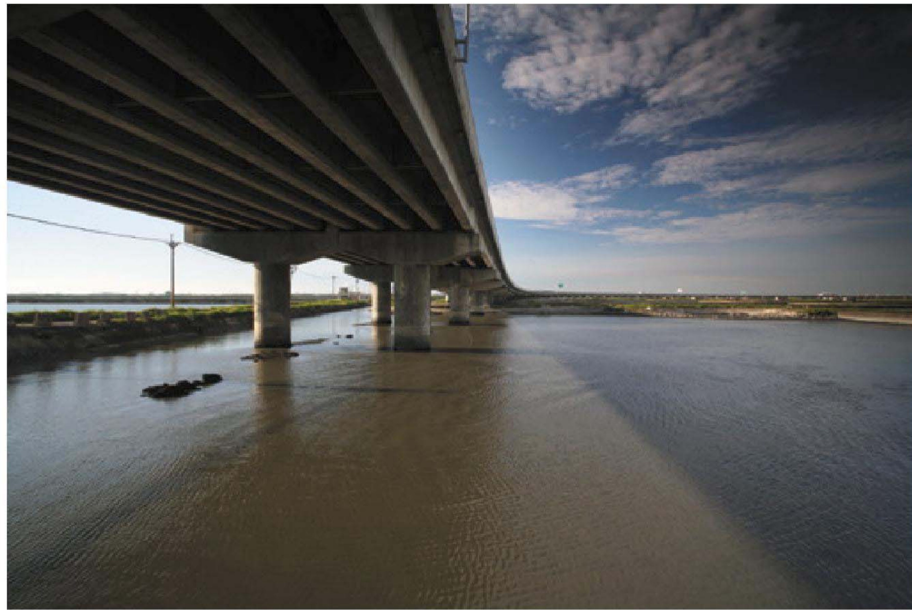
臺61線232K高架橋下 Taiwan Provincial Highway No.61 at 232K beneath the viaduct
