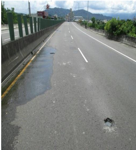
Fig. 1 Pothole (taken by DGH)
