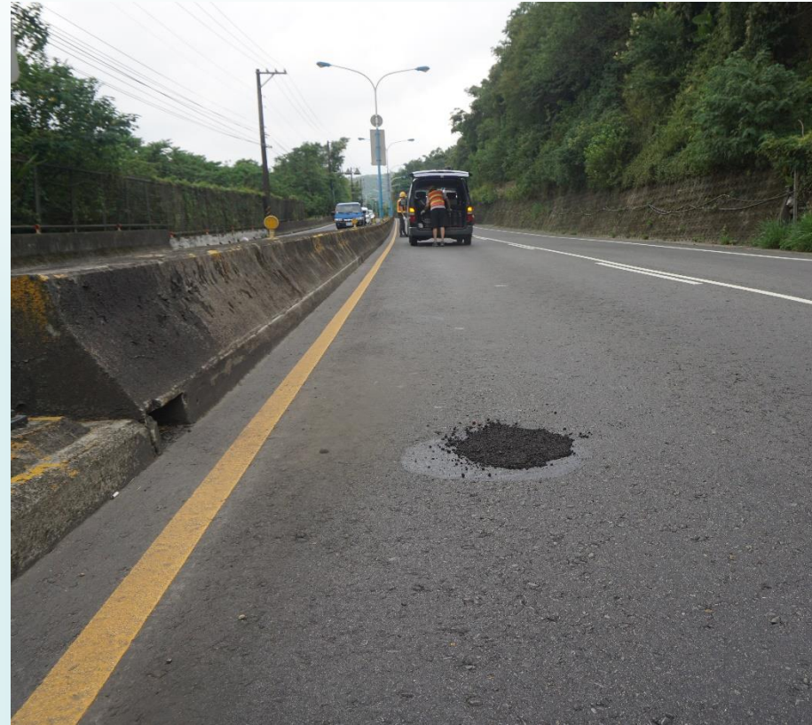
Example of poor patching (Photo taken by DGH)
