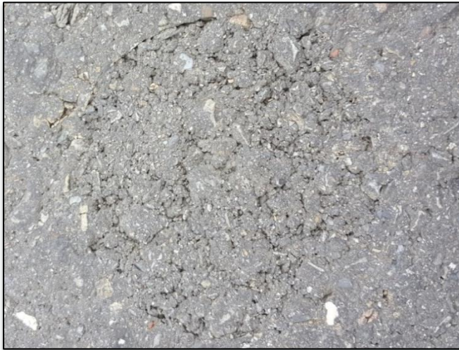
Regular patching materials (After four months)
