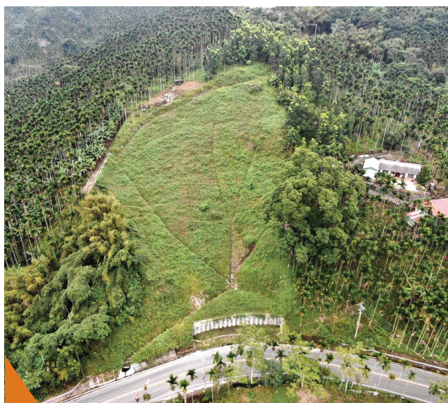
台18線41k+100左側坍塌修復施工後。 Repair completed for the left side slope on the section of 41k+100 of Provincial Highway No.18.
