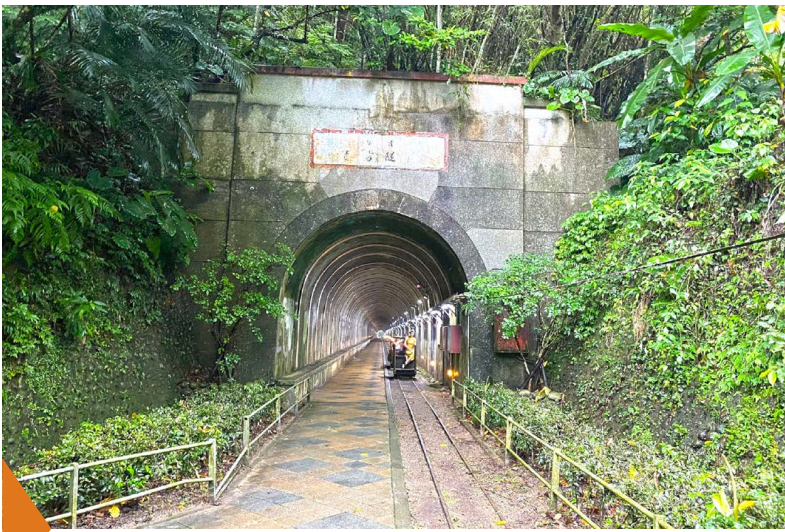
台7線7.7k活化舊百吉隧道。 Restored Old Baiji Tunnel at 7.7k of Provincial Highway No.7.
