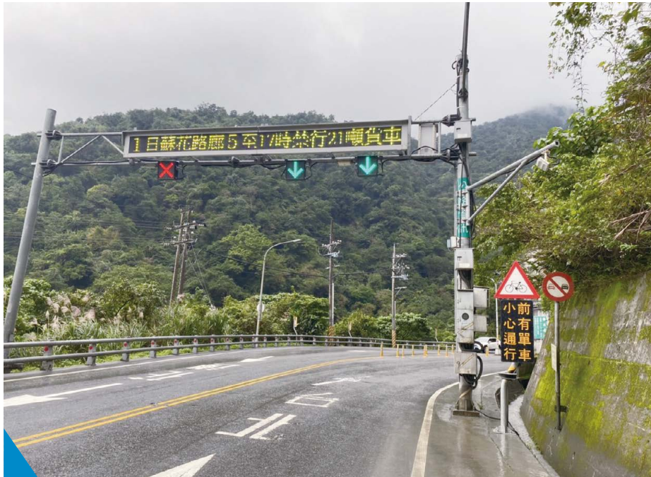
新澳隧道南口告警系統。 Xin'ao Tunnel south exit alert system.
