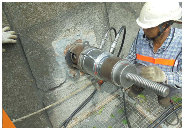
台14線42k+050地錨揚起試驗，檢查地錨拉力足夠。 Earth anchor lift-off testing for the section of 42k+050 of Provincial Highway No.14 to ensure sufficient tension.
