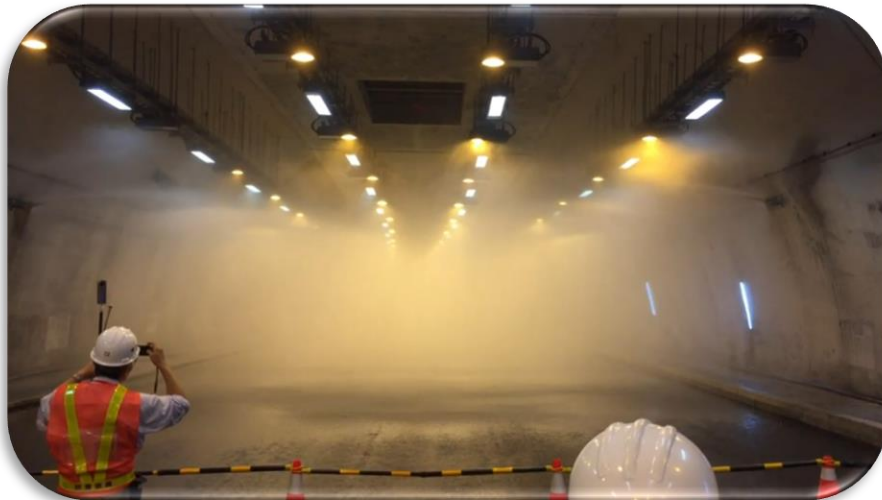
Figure 2-8 Picture Showing Cooling of Tunnel by Water Mist Spraying in Tunnel
